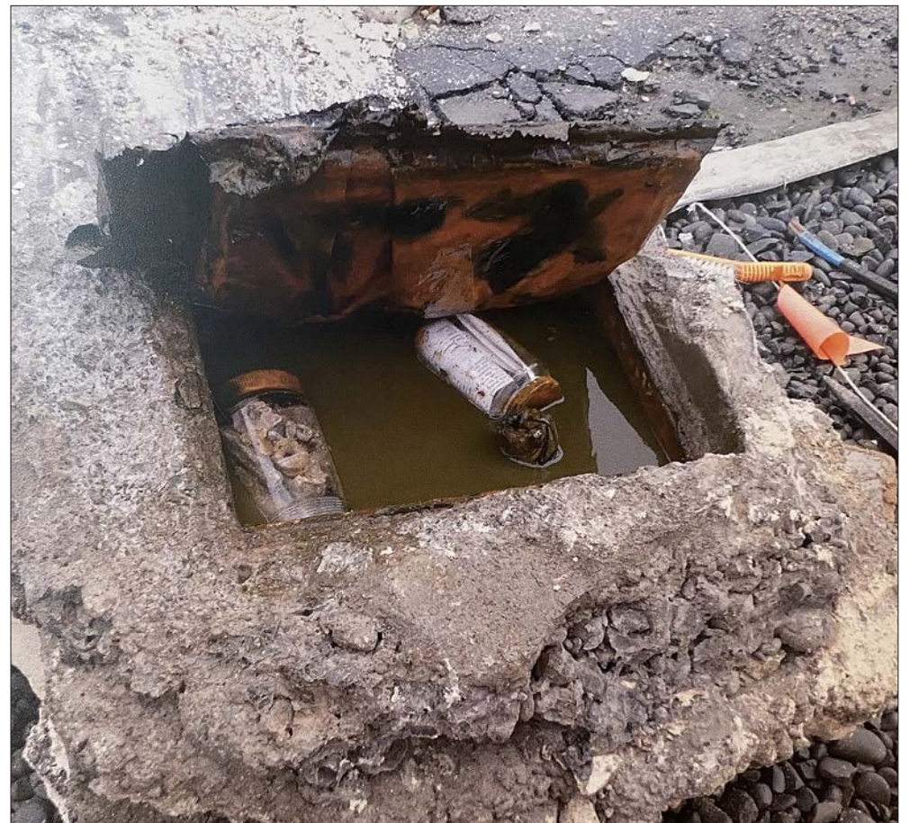
The box containing two coffee jars uncovered after the demolition of the Cathedral of the Blessed Sacrament
